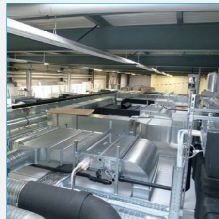
Air conditioning and circulation units
